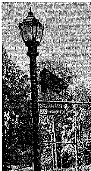
Solar & Existing Pole
